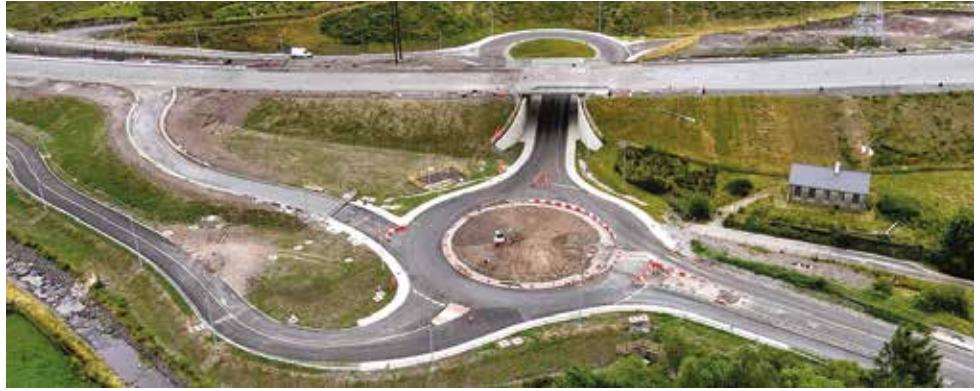
New road layout at the western end of Ballymakeera, as the Macroom Ballyvourney Bypass nears completion. © Peter Scanlan
