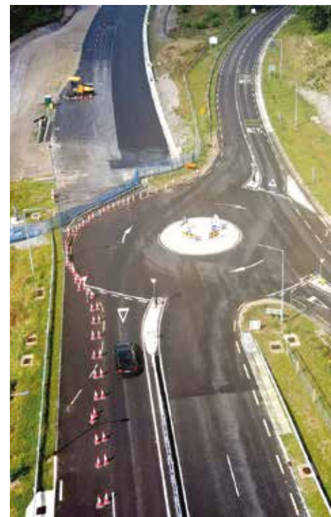
Temporary Roundabout at Carrigaphooa Castle due to be removed, as the Macroom Ballyvourney Bypass nears completion. © Peter Scanlan
