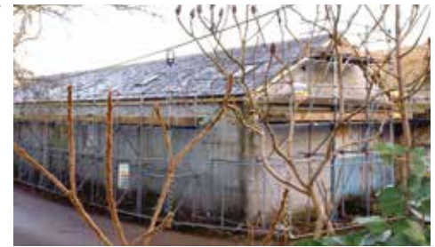
Macroom Bus Station and former Railway Station (and currently being roofed and refurbished) (C. Kelleher.).
