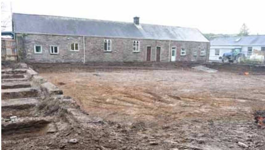
Site of Macroom Community Hospital extension with exposed structure from Macroom Workhouse times
