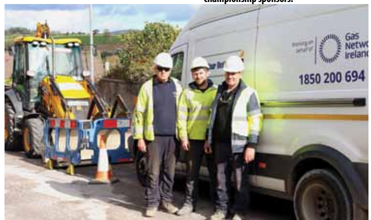
Gas men installing gas pipes for the five new houses in Oakwood. Con Moynihan, Toonsbridge, Steven O'Leary and Chris O'Leary Ballinagree. (Con Kelleher)
